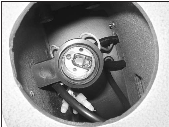
Figure 56. Light socket with dust plug removed (for 120V operation only).
