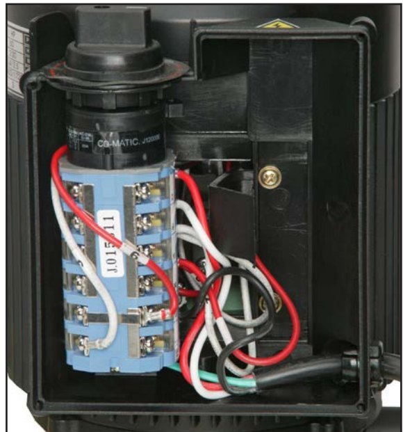
Figure 28. Motor switch (front view, G1096).
