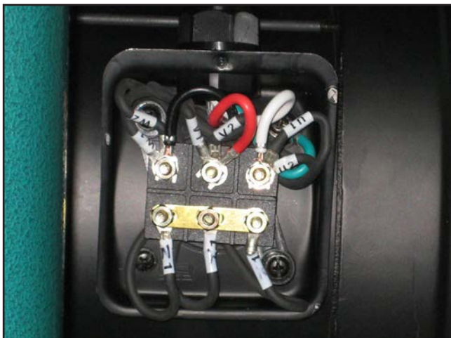
Figure 156. G0606X1/G0697X motor junction box.
