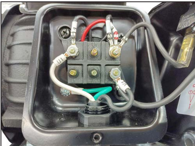
Figure 107. Motor junction box wiring.
