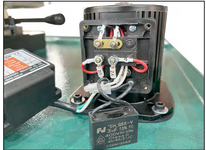
Figure 1. Pump motor wiring.
