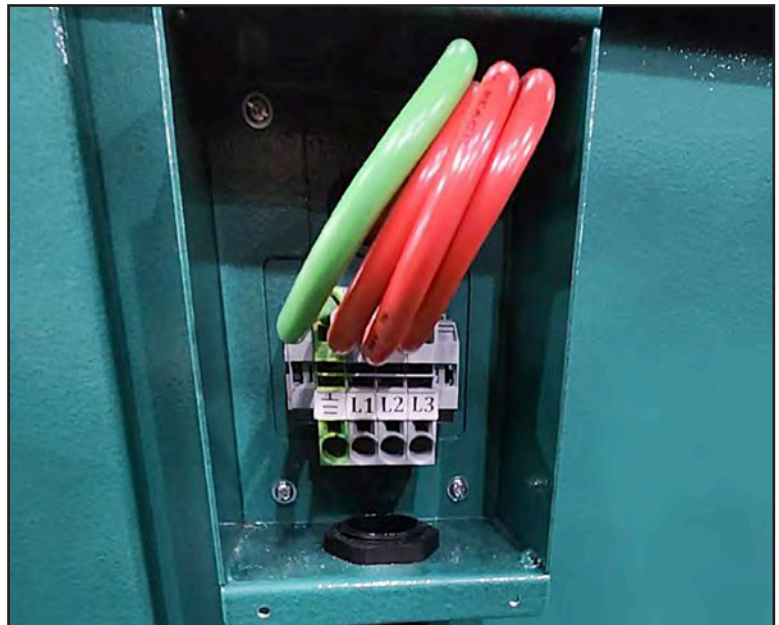
Figure 86. G0450 power junction box.
