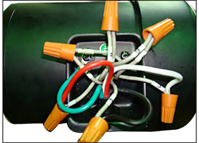
Figure 98. G0450 480V feed drum motor wiring.
