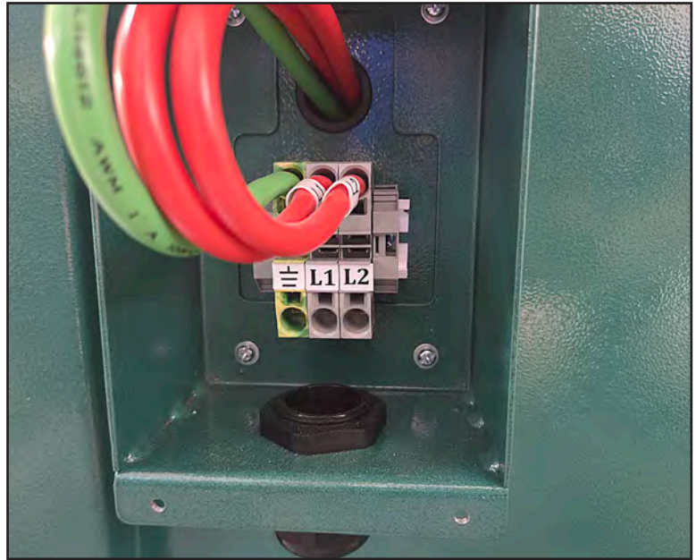
Figure 85. G0449 power junction box.
