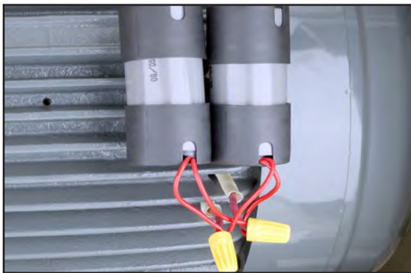
Figure 90. G0449 sanding drum motor run capacitors.
